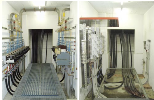
Figure 6 Low voltage electric board before and after modifications.
